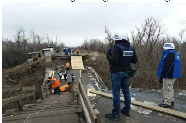
Repairs to Stanytsia Luhanska bridge wooden ramps, Luhansk region on 9 December 2017. (OSCE)
