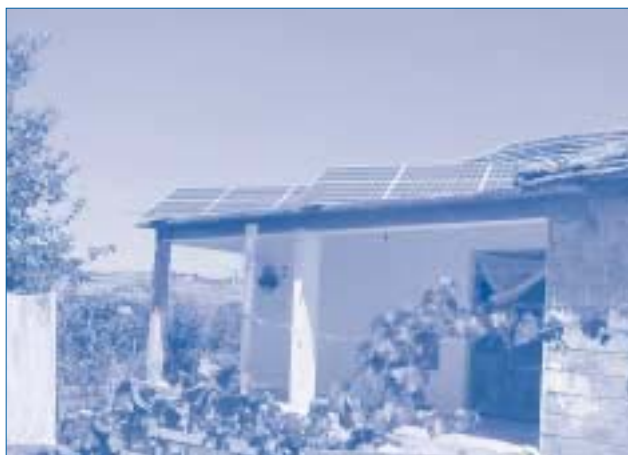
Photovoltaic panels installed on Hysgjokaj village, Albania
