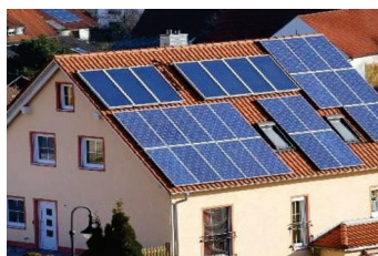
Rooftop PV system
