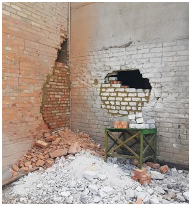
Damaged wall of the main building of the water pumping station in Kyivskiy District of Donetsk being repaired, May 2021.
