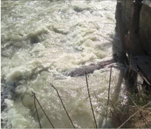
Picture 13: Outdoor water intake facility of from perforated pipes
