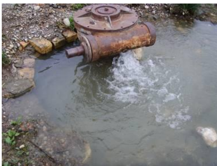
Picture 12: Section in critical condition on water pipeline between Points 3 and 4.
