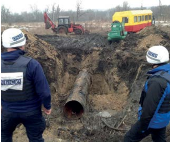
OSCE SMM monitors observing and facilitating repairs to water pipelines near Artema, Luhansk region, 11 January 2017. (OSCE/Igor Danis)
