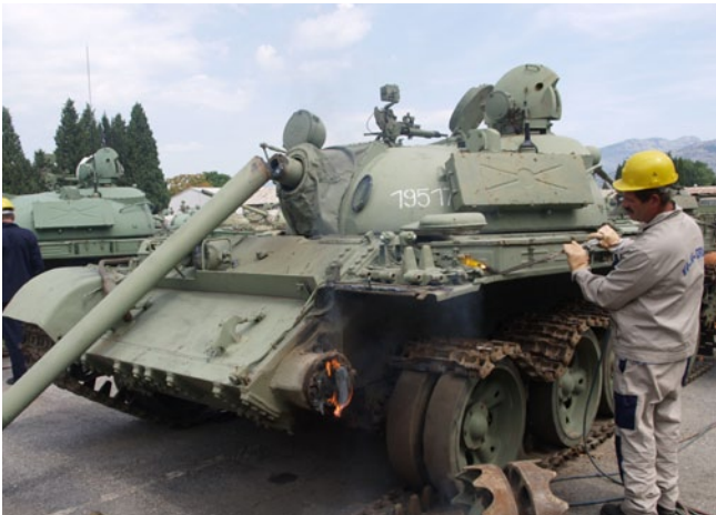
T-55 tank being melted for scrap and recycled as part of the MONDEM Demilitarization Programme. Credit: MONDEM Programme
