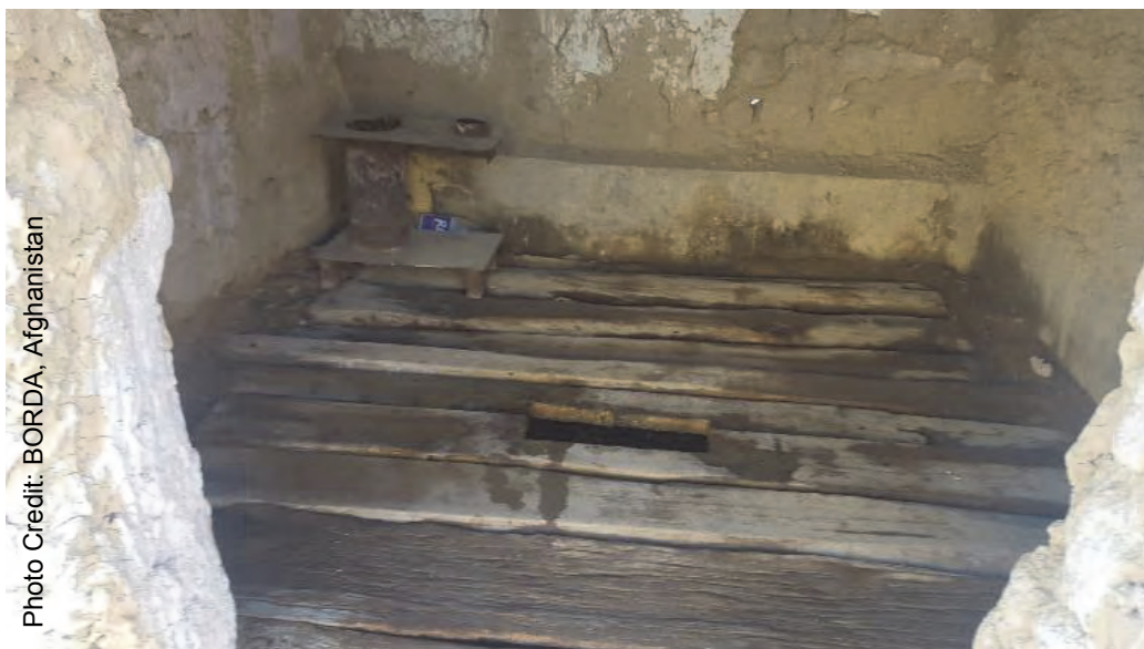
FIGURE 7. TOILET WITH WOODEN PLANKS AS COVER
