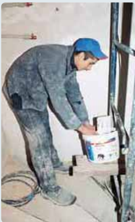
Orphan Eugene Diduk at work as a plasterer at the construction site of the new Kharkiv entertainment centre.
