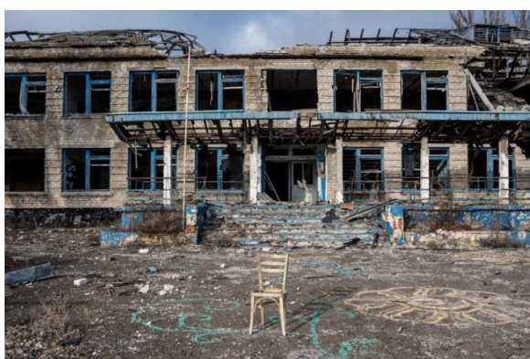
School in Shyrokyne damaged by shelling in 2015
