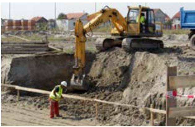
Construction works in Ovca, Serbia, which is the biggest RHP construction site in the region, 9 September 2016 (OSCE/Milan Obradovic)
