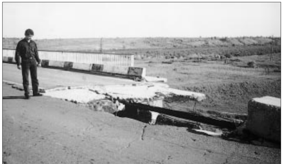
The damaged Gura-Biculi bridge over the Dniester river
