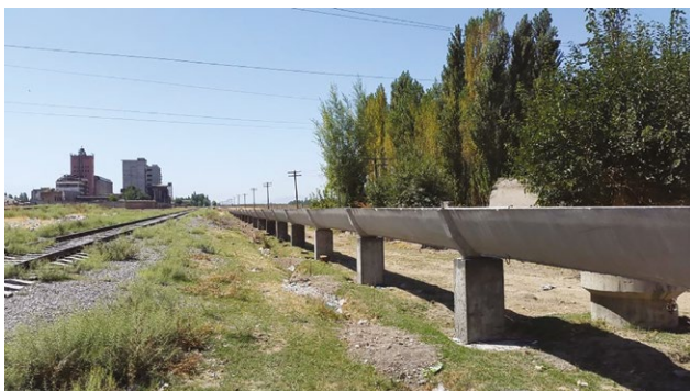
The OSCE Centre in Bishkek and local authorities rehabilitated the Kara-Suu canal, easing disputes with communities across the Uzbek border over irrigation water
